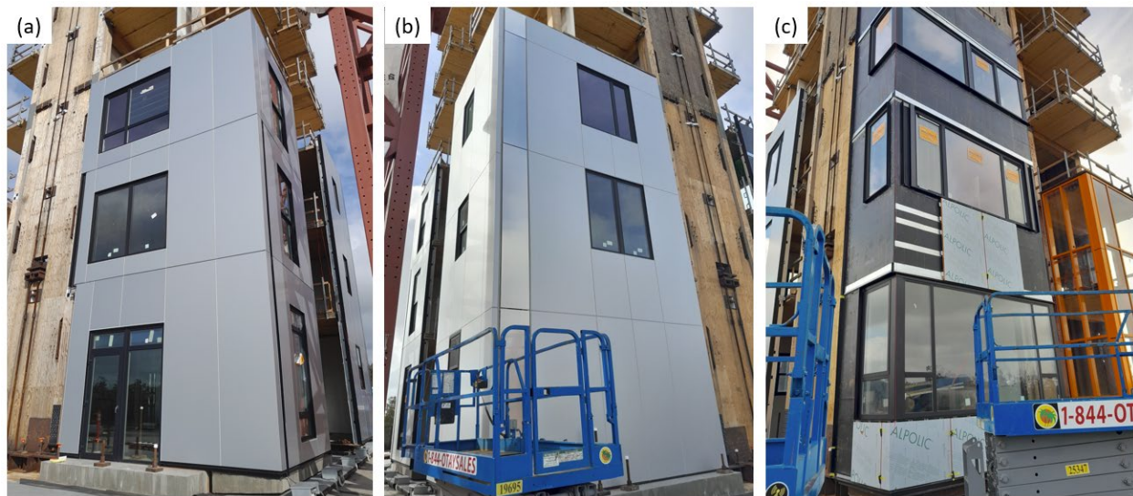
Figure 1: (a) Completed platform-framed subassembly (CFS 1), (b) completed bypass framed subassembly (CFS 2), (c) spandrel framing subassembly in final stages (CFS 3).
